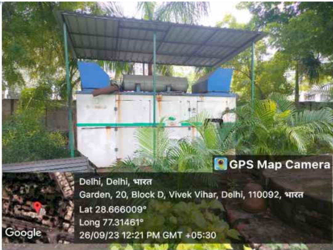
Figure 20. Soundproof silent generators
